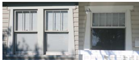
3/1 and 5/1 double hung sash windows Battered casing surrounding windows
